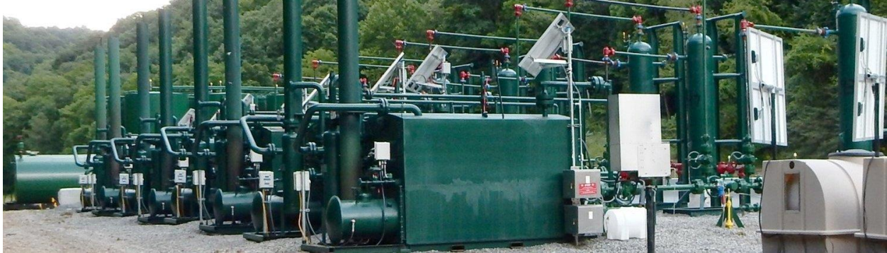
Figure 11 Gas well GPU's on a shale well pad
